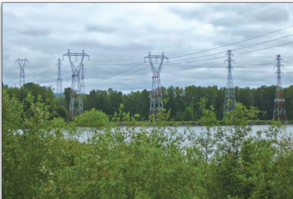
BPA's river-crossing towers in Longview, Wash. The voltages are 115kv, 230kv, and 500kv, and the tallest one is approximately 460 feet.
