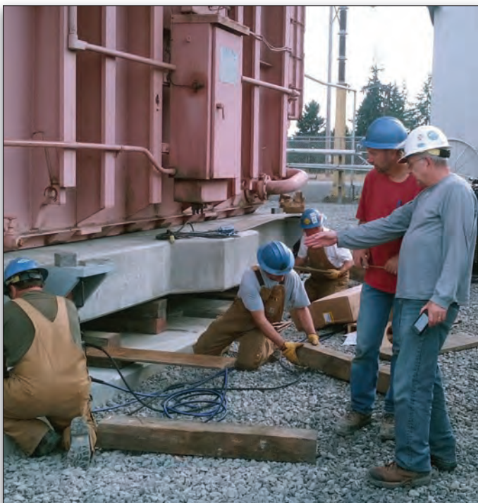
Seismic Program Manager Leon Kempner and Electrical Rigger Foreman II Rick Wiren discuss how to install the base isolators on the 400,000-pound transformer.
